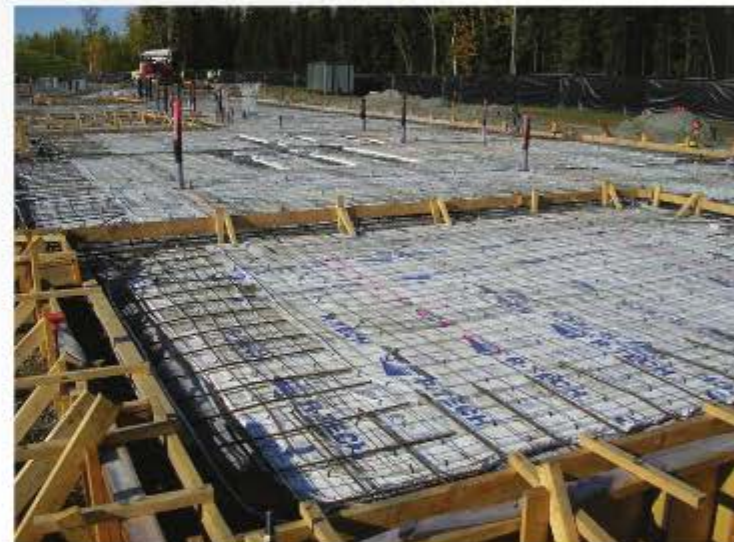
INSULATION was installed both vertically and horizontally to trap heat below the slab and keep the soil underneath thawed despite at-times freezing temperatures.
