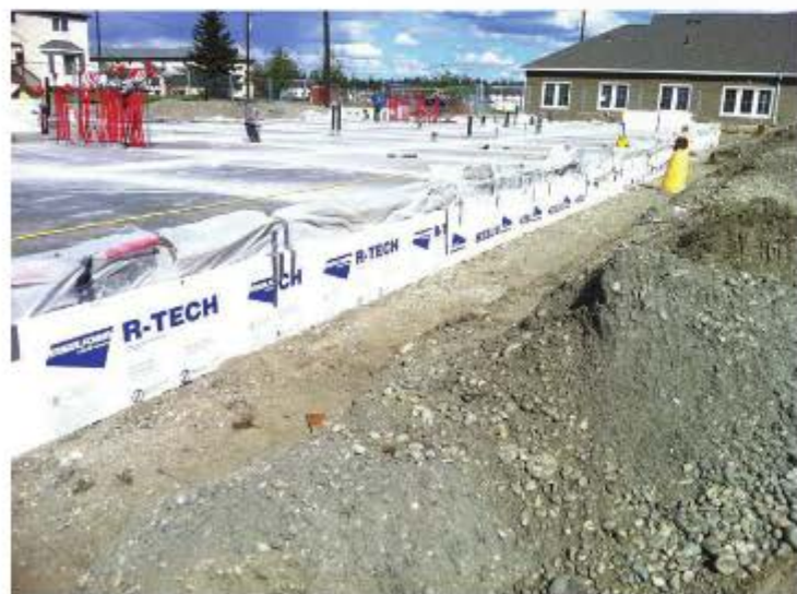
EPS INSULATION was installed below the slab on a 275-unit military housing project in Alaska. (All photos of courtesy Insulfoam)
